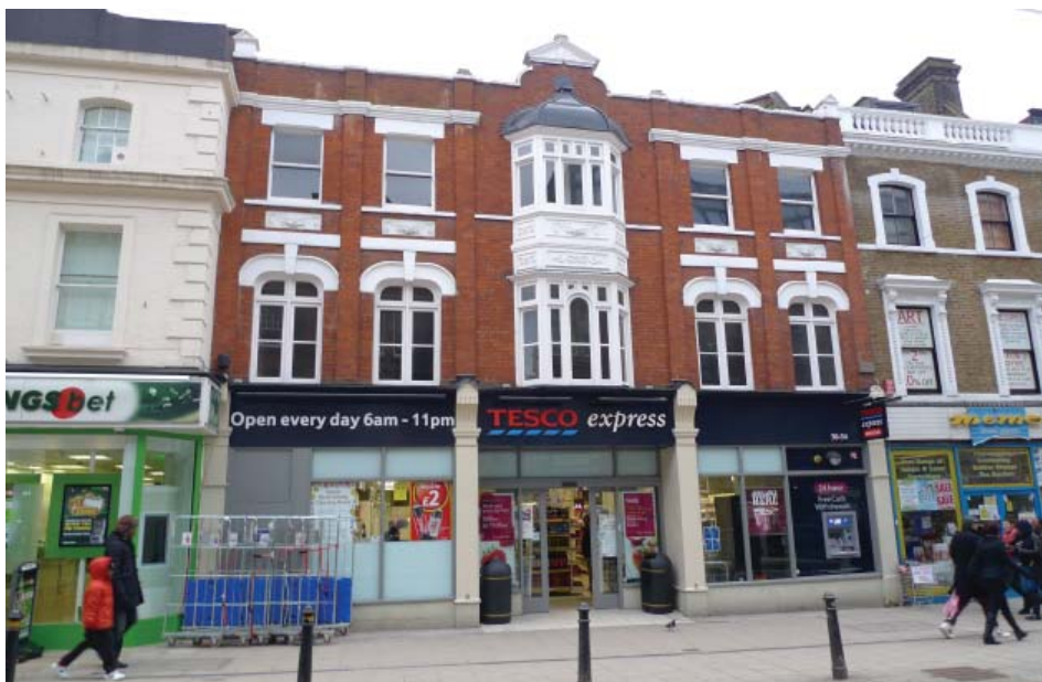
Recently restored and cleaned facade on George Street that has enhanced the appearance of the building and the wider conservation area
