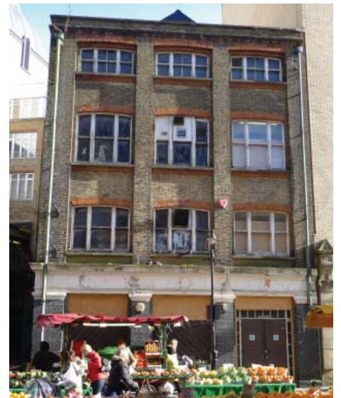
46 Surrey Street, the former Croydon Advertiser building, is currently in a poor condition
