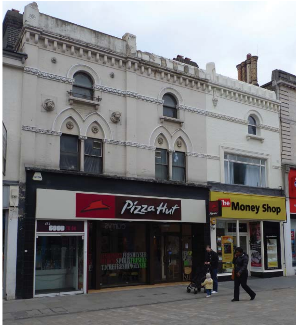
57-69 North End, locally listed. Unsympathetic window replacement and alteration to the window opening (above right) and a modern shop front and oversized fascia that disregards the character of the architecture above (above left)
