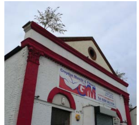
Vegetation in the gutter at 47 Tamworth Road, showing neglect and a lack of maintenance
