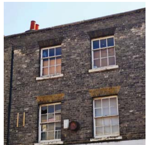
Poorly maintained timber sash windows and cills
