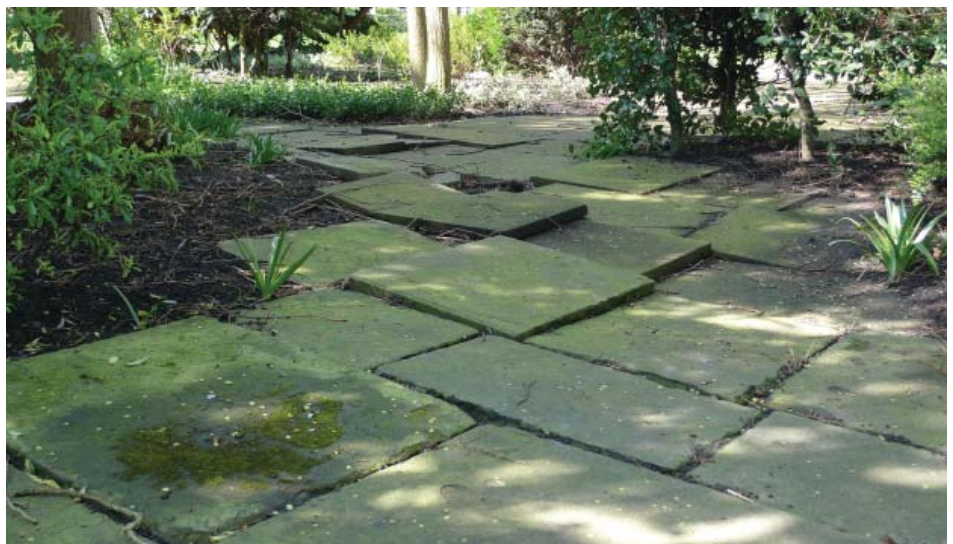
Tree root or damage from vandalism at St John's Memorial Garden
