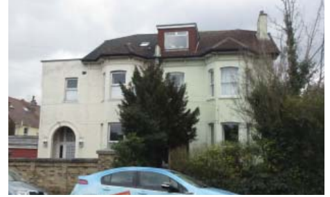
Poor quality extensions to a building on Havelock Road - the side extension is not set back from the front wall of the house and does not respect the building's character and design and the roof extension is oversized and of an insensitive design.
