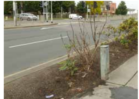
Guardrail, landscaping in poor condition and patched footways do not create an attractive pedestrian environment along Roman Way
