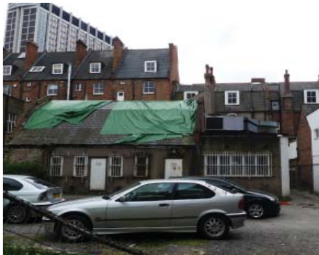
The rear of George Street is poorly maintained
