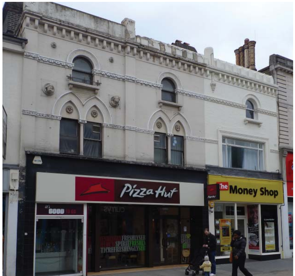
57-61 North End, locally listed. Unsympathetic window replacement and alteration to the window opening (above right) and a modern shop front and oversized fascia that disregards the character of the architecture above (above left)
