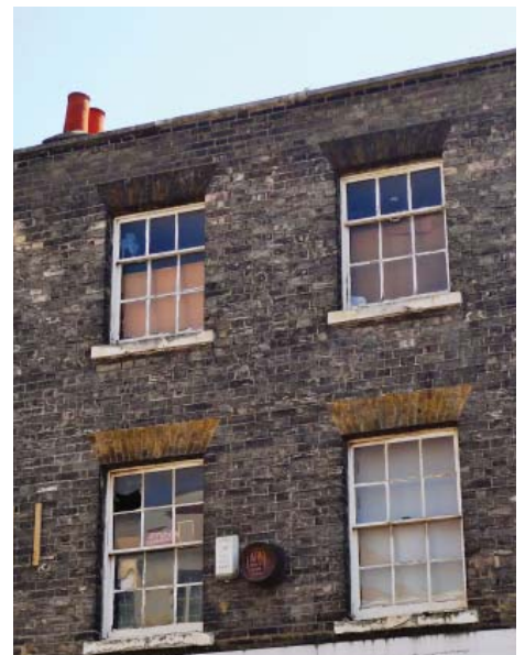
Poorly maintained timber sash windows and cills
