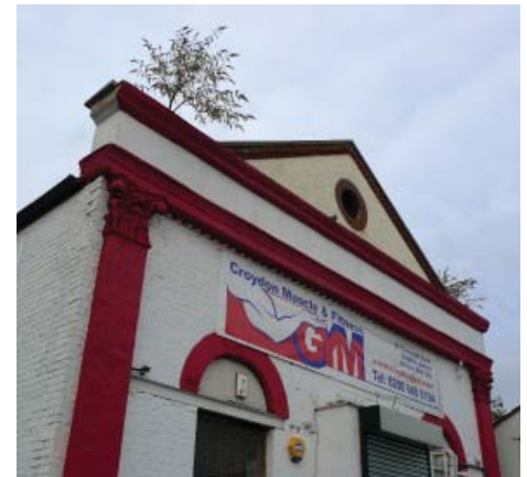
Vegetation in the gutter at 47 Tamworth Road, showing neglect and a lack of maintenance
