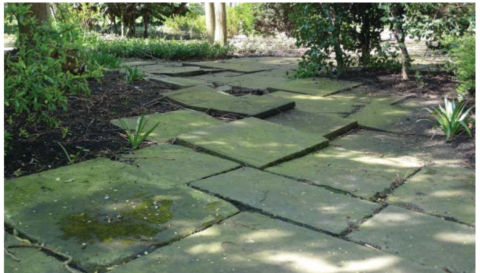
Damage to paving stones at St John's Memorial Garden
