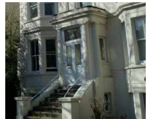
Originally an open porch with free standing columns and infill that has been enclosed, harming the appearance of the property
