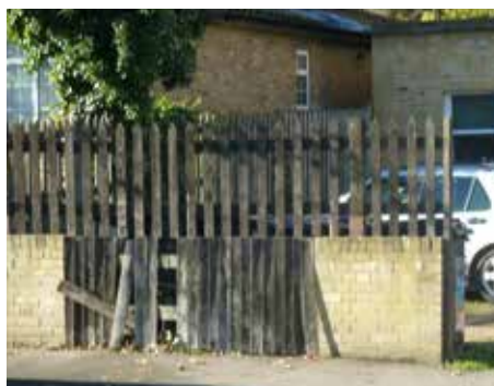
Poor repair to boundary wall
