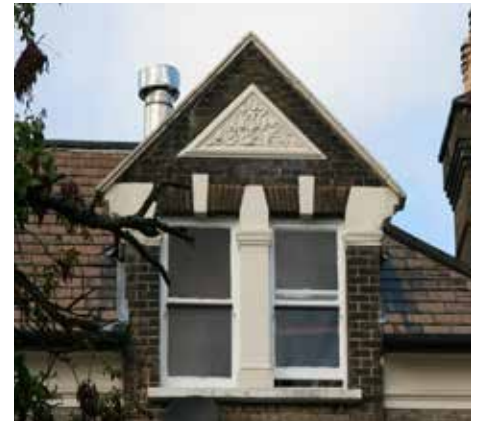
Visible flue from the streetscape
