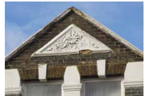
Historic plasterwork in need of repair
