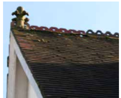
Poor repair of decorative roof tile
