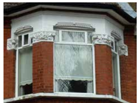
Replacement of original windows for uPVC windows. Proportions and material are unsympathetic
