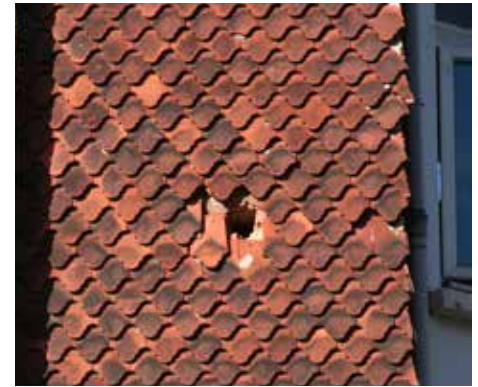
Hanging tiles in need of repair
