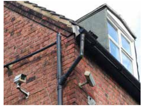
Poorly sited CCTV and unsympathetic dormer.
