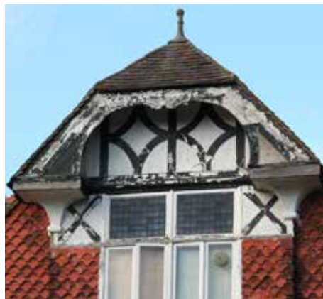
Poorly maintained timber bargeboard
